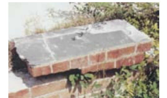
The image above shows a thin layer of slate used as a damp-course to prevent the upward movement of moisture.
